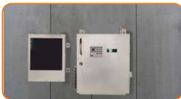
COD Server Ethernet Switch TCU
