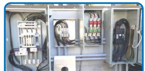
Electric Control System
